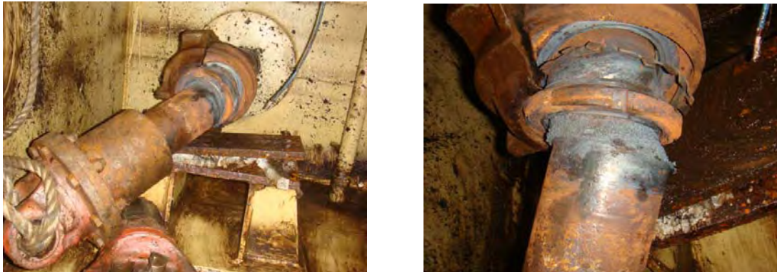
Fig. 1.3 Destroyed high speed shaft line with cardan shafts
